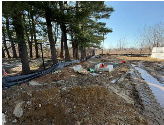
Picture 7: Silt Fence (S)
