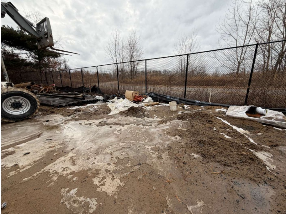
Picture 1: Section of Silt Fence in Disrepair
