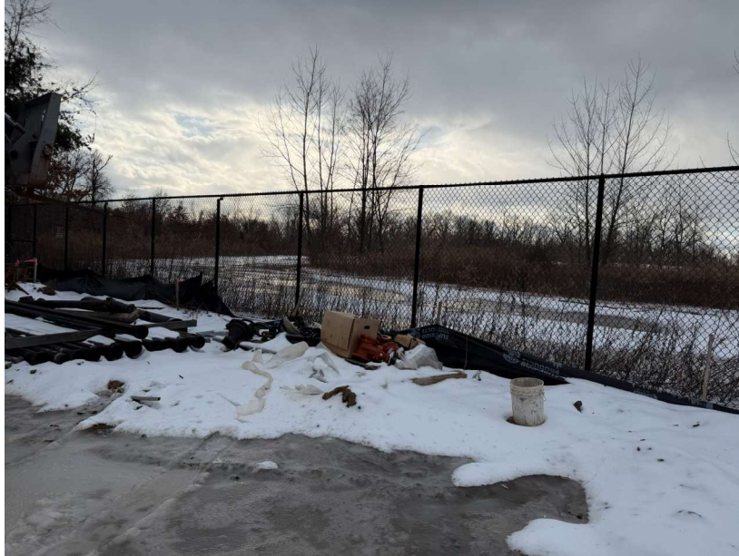
Picture 1: Section of Silt Fence in Disrepair
