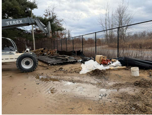
Picture 1: Section of Silt Fence in Disrepair
