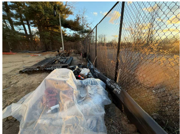
Picture 4: Section of Silt Fence in Disrepair
