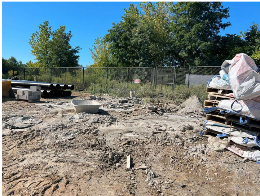
Picture 2: Remnants of Concrete Washout Area
