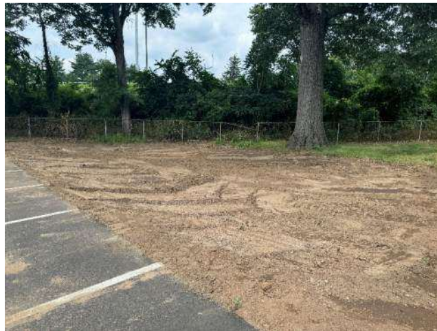
Picture 2: Soil stockpile area has been removed. Seed and stabilize area if no longer in use.
