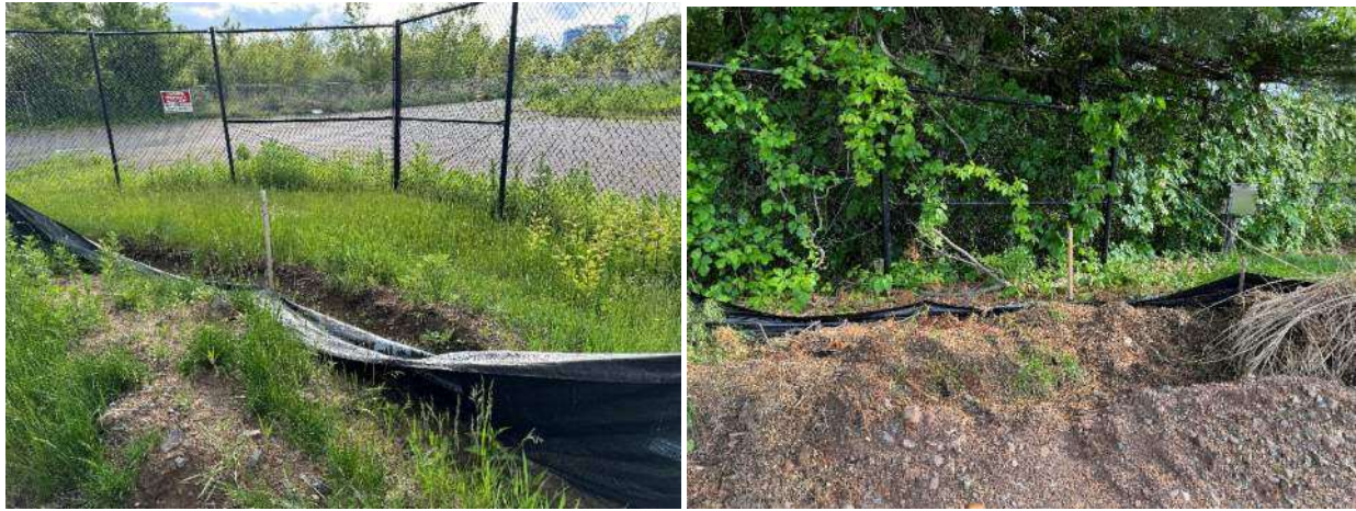
Picture 7 & 8: Silt fence needs to be reattached to stake along project edge.
