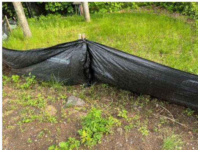
Picture 6: Silt fence not buried.
