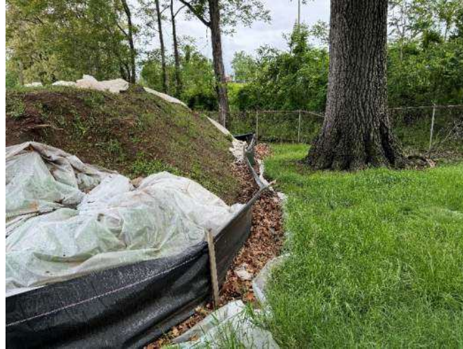
Picture 1: Silt Fence post down around stockpile area.
