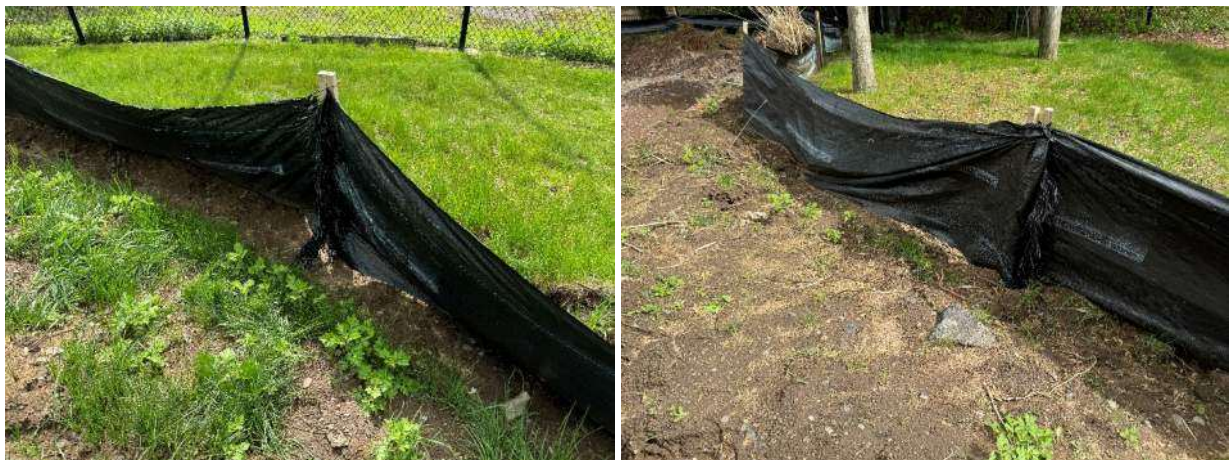
Picture 5: Silt fence not buried.
