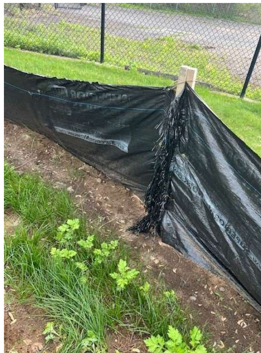
Picture 3: Silt fence not buried.
