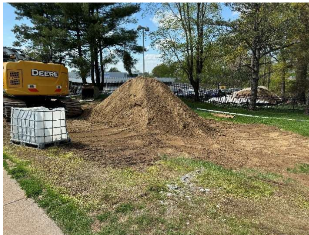
Picture 2: Stockpile area/disturbed area needs silt fence.
