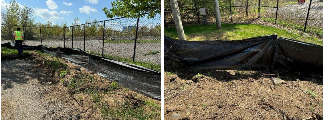
Picture 5: Silt fence not buried.
